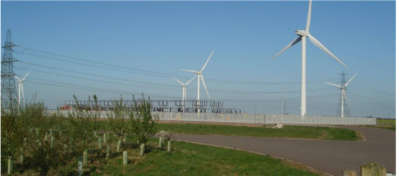
Image 3.2 Existing Bicker Fen 400 kV Substation (Source: National Grid)
