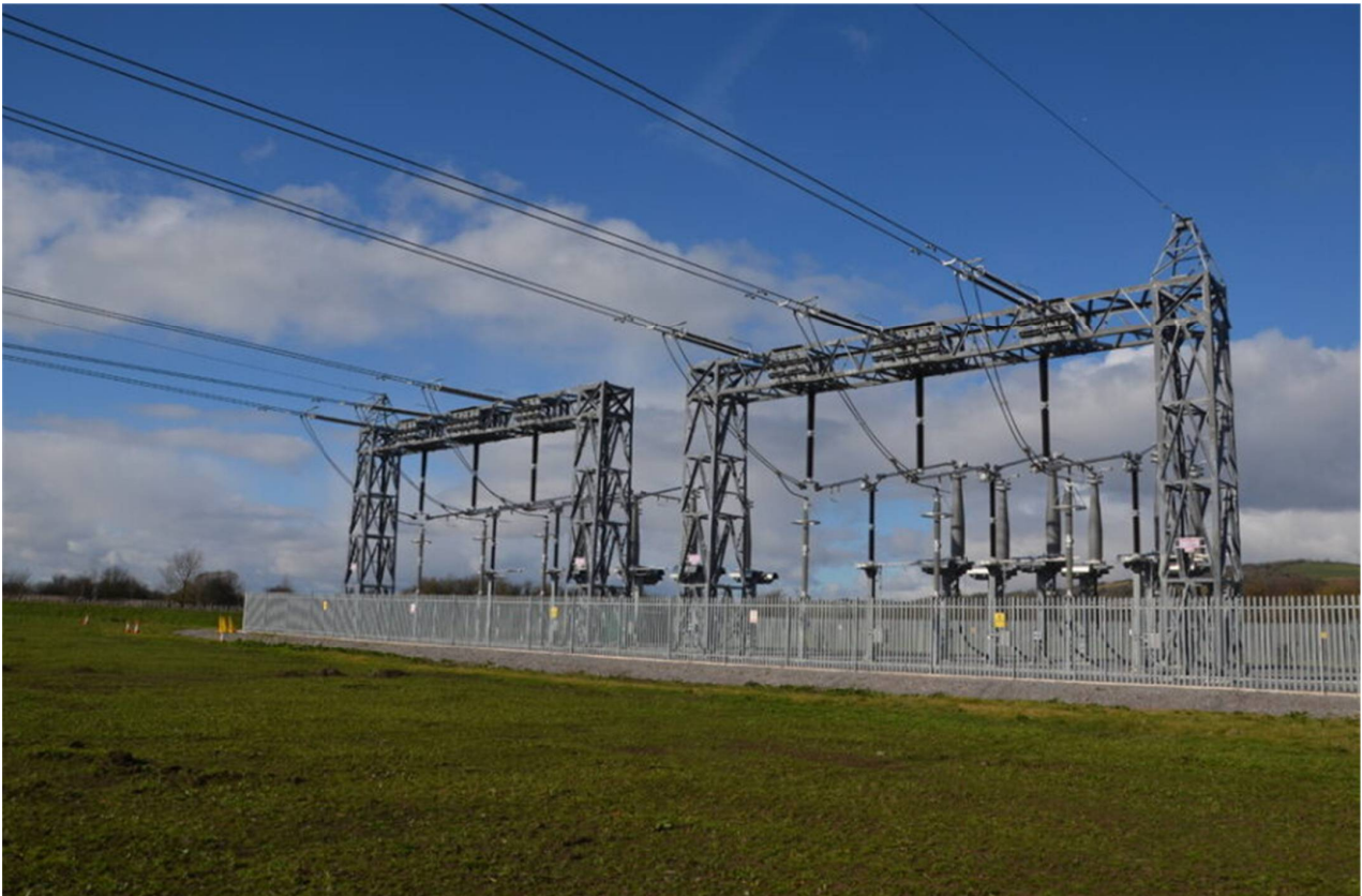
Image 3.9 Existing CSE compound with gantries (Source: ES Chapter 4: Project Description (document reference 6.4[APP-130]))
